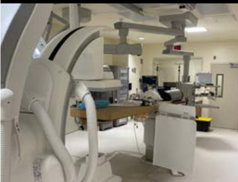
W. W. Gay Mechanical Contractor, Inc. Ascension St. Vincent's Clay County Cath Lab Expansion Phase 3 Jacksonville, FL
