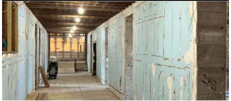
Ponce De Leon Hall East Wing Renovations W. W. Gay Mechanical Contractor, Inc. Saint Augustine, FL
