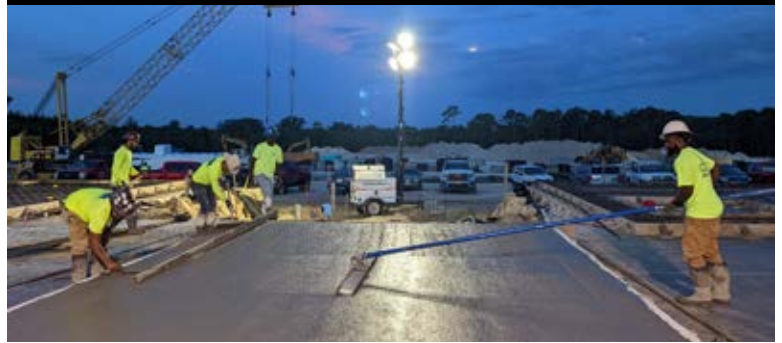
Imeson Landing Business Park (Phase II) A.A. Pittman & Sons Concrete Jacksonville, FL
